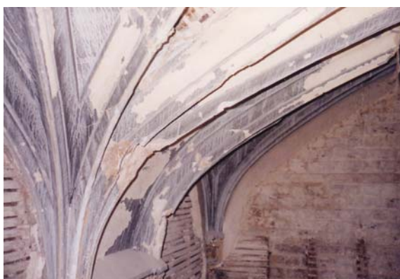
Pictured above is one of fluted ribs in the Equerries Staircase at Windsor Castle which Hayles and Howe restored after the disastrous fire in 1995. The Lime works completed here won Hayles and Howe a regional award from the FPDC in 1998.
